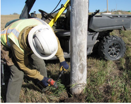
Pole testing reduces pole failures and improves system reliability.
